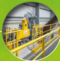
2019 The Erden- & Substratwerk Tabeling is building a new production and storage hall
